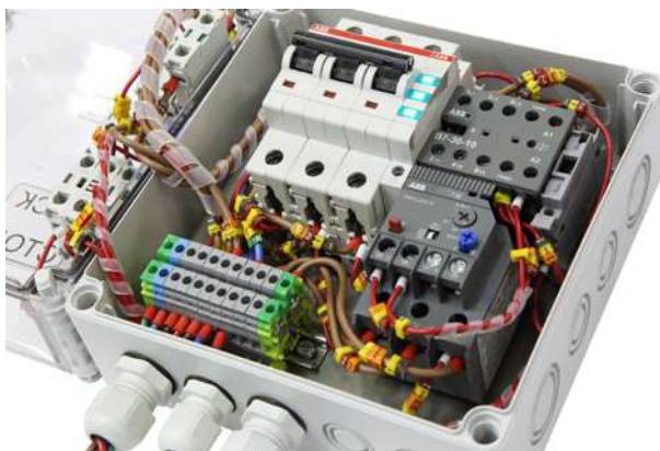
PCP3 control panel
